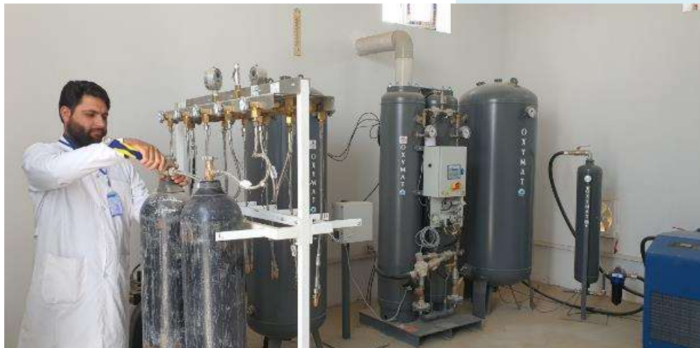
Oxygen plant in Nimroze
